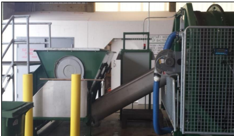
Figure 52. The Enviro-Drum at WDOC's Cedar Creek Facility.
