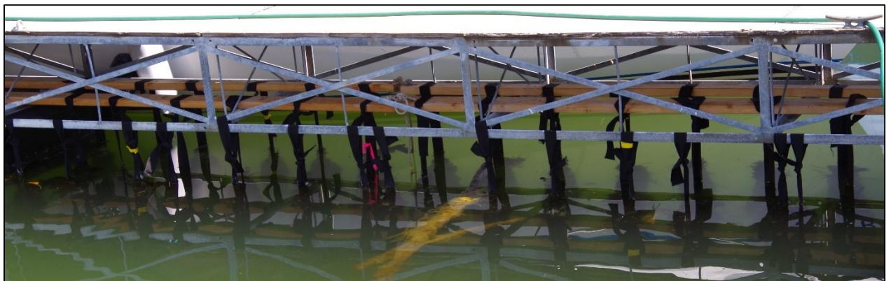
Figure 4. Straps affixed to dock at West Bay Marina, Budd Inlet.
