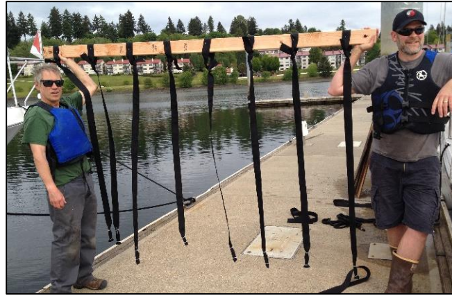
Figure 5. Nylon straps prior to being affixed to the dock at Boatworks, East Bay.
