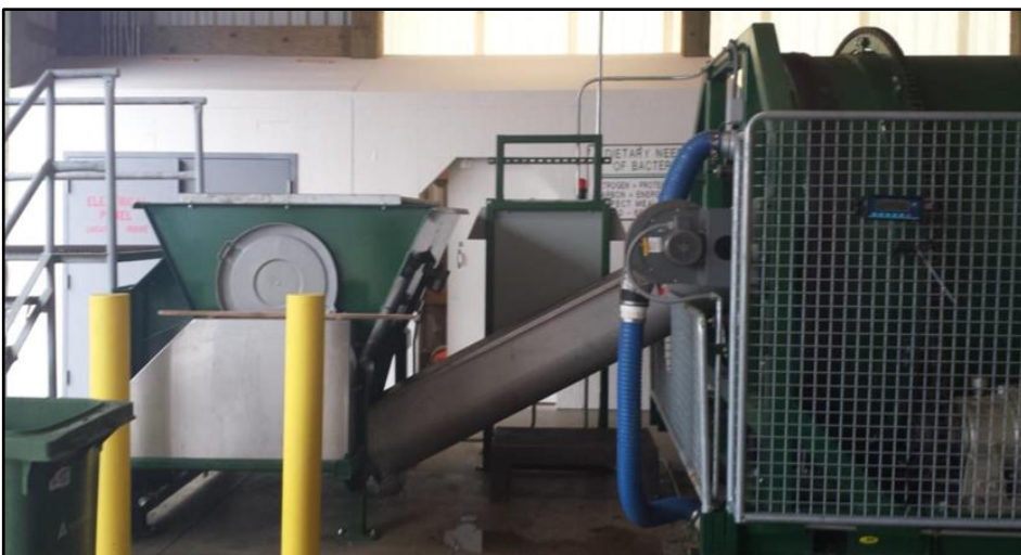
Figure 10. WDOC's Earth Drum composting system by DT Environmental
